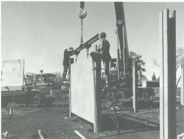
Workmen slot a pre-cast concrete panel into concrete pillars during the early stages of a house under construction.
